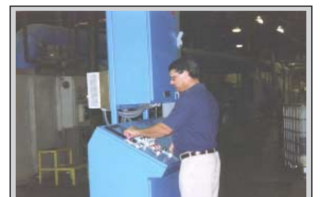
RMax's hydrocarbon injection system main control panel
