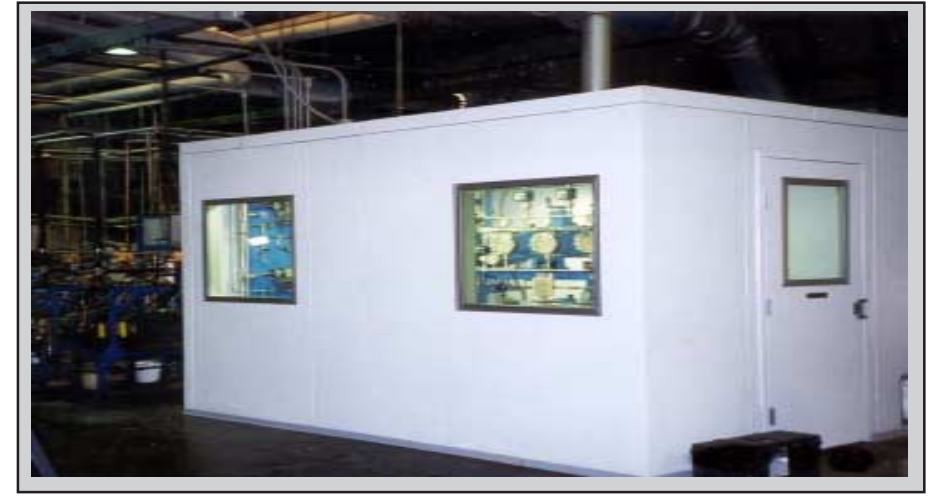
RMax's ventilated enclosure surrounding its high pressure injection pumps
