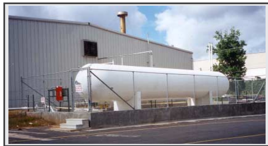
RMax's 12,000 gallon Hydrocarbon Blowing Agent storage tank
